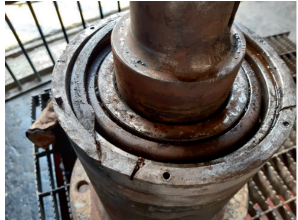
Fig. 4. Wear found at the base of the lower bearing.
