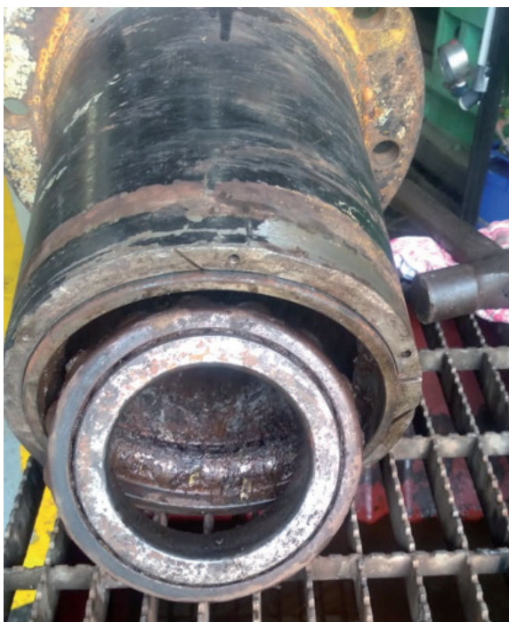
Fig. 3. Lower bearing of the jib crane bracket.
